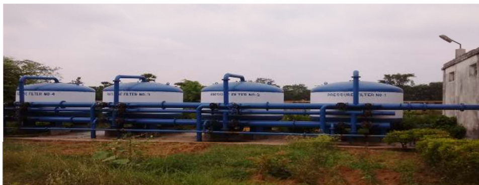
Pressure Filters at the Gangajalghati WTP
