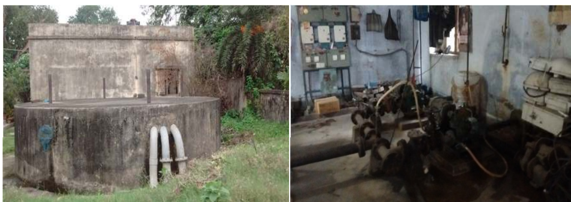
Existing ground level reservoir and pump house
