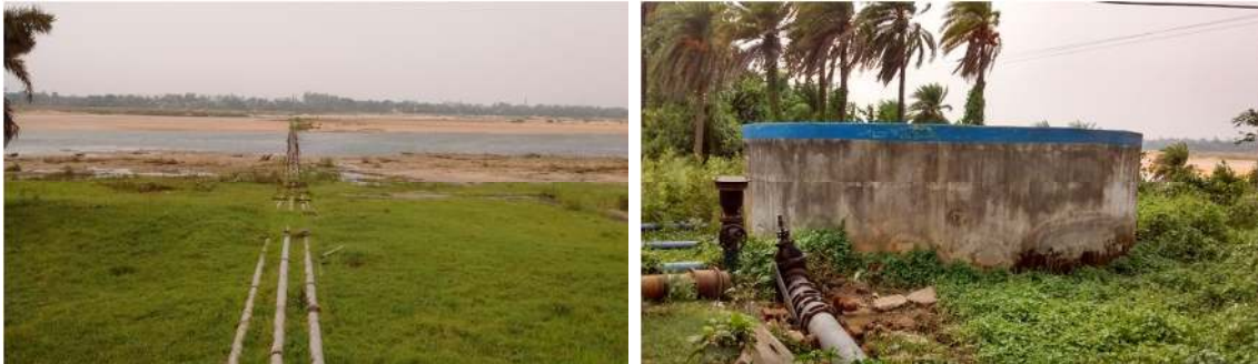
River bed tube wells and the ground storage reservoir
