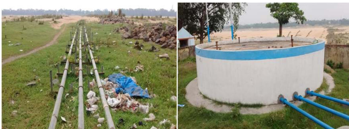
Raw water mains from river bed tube wells and the new reservoir
